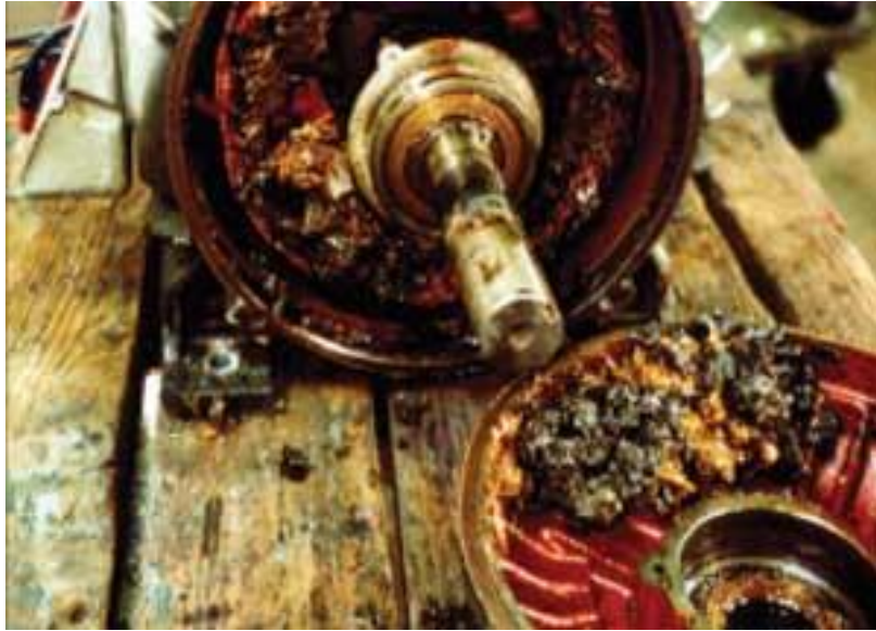
Figure 8. Overgreasing caused inside of motor to fill with grease.
